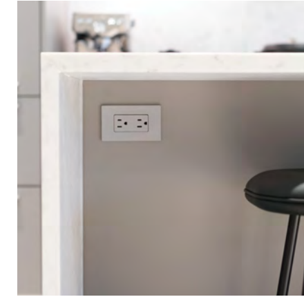
Multiple outlets integrated in the island
